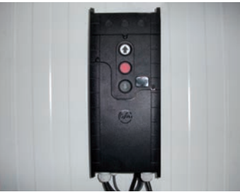
Control panel for cold room rapid door.
